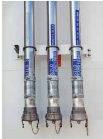
Truck fill lines
